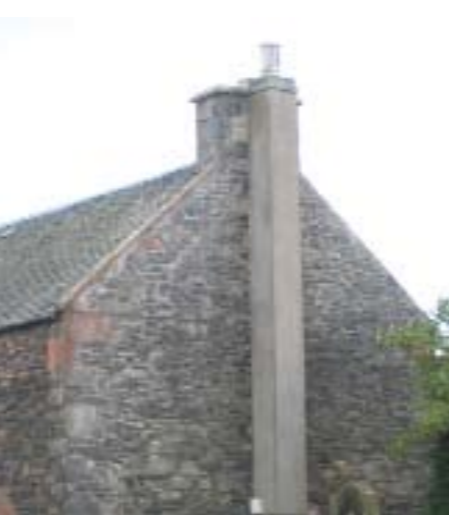
A new flue on the outside face of the gable
