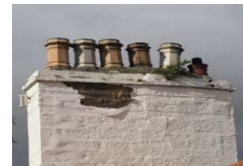
A mid 19th C chimney and cans showing a variety of problems.
